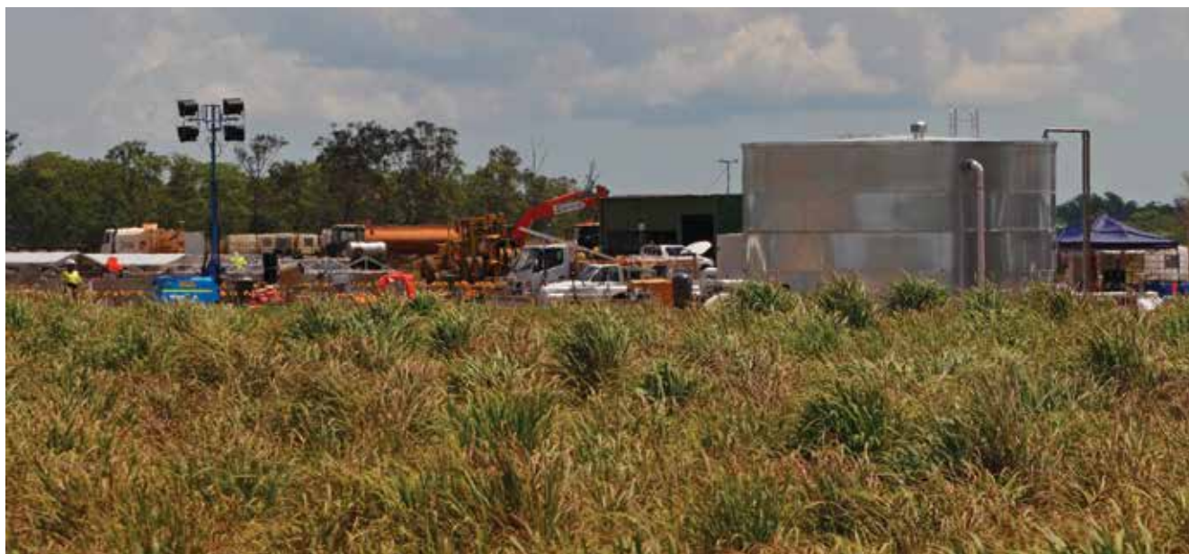
Image: Construction of the new crocodile farm at Lambells Lagoon, Northern Territory.
